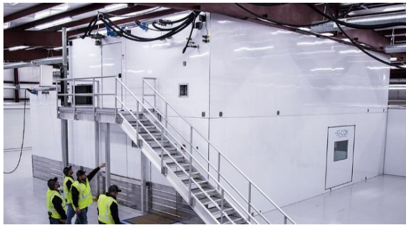
G-CON's autonomous, cleanroom POD
