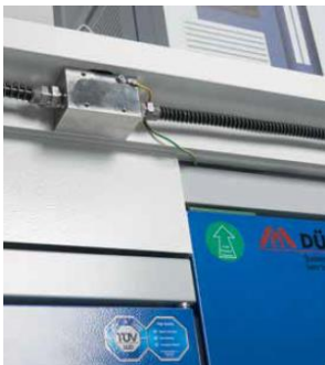
Connection to earthing and T-distributor made of stainless steel
